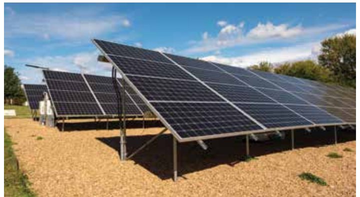
Solar arrays are present at and help power many of our centers, including the one above in Wichita.
